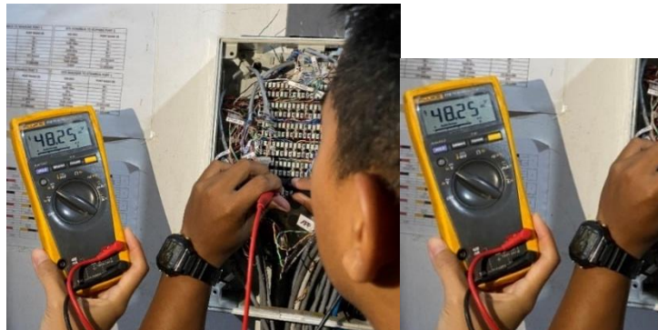
Gambar 3. Pengecekan Tegangan Box MDF Main
